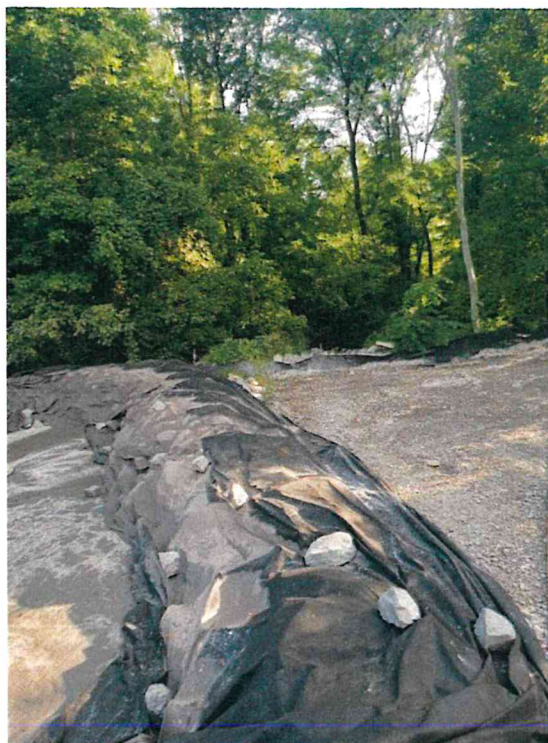
June 22 - Manhole 1750 Before Cleanup
