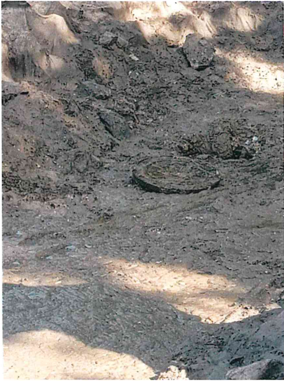
June 11 - Manhole 1750 Before cleanup
