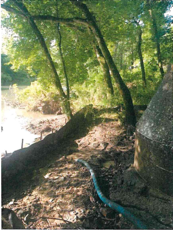
June 11 - Manhole 1748 Before cleanup
