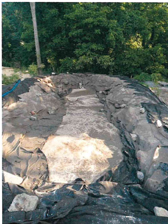
June 22 - Manhole 1750 Before cleanup
