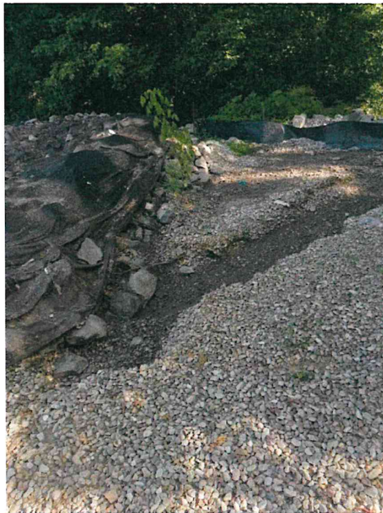
June 11 - Manhole 1750 Before cleanup
