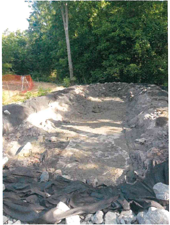
June 11 - Manhole 1750 Before Cleanup
