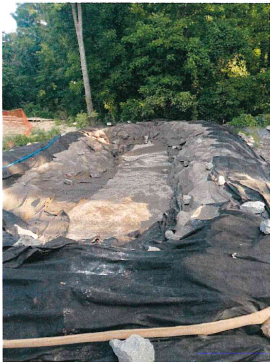
June 22 - Manhole 1750 Before cleanup
